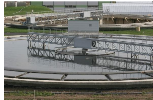
Restoring the ecological health of the Baltic Sea. Southwest Wastewater Treatment Plant in St. Petersburg, Russia.
